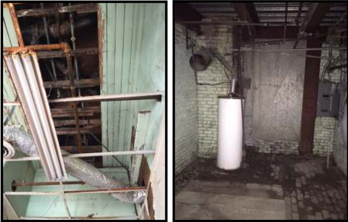
(L) Original plumbing with signs of corrosion (R) Missing boiler in basement
