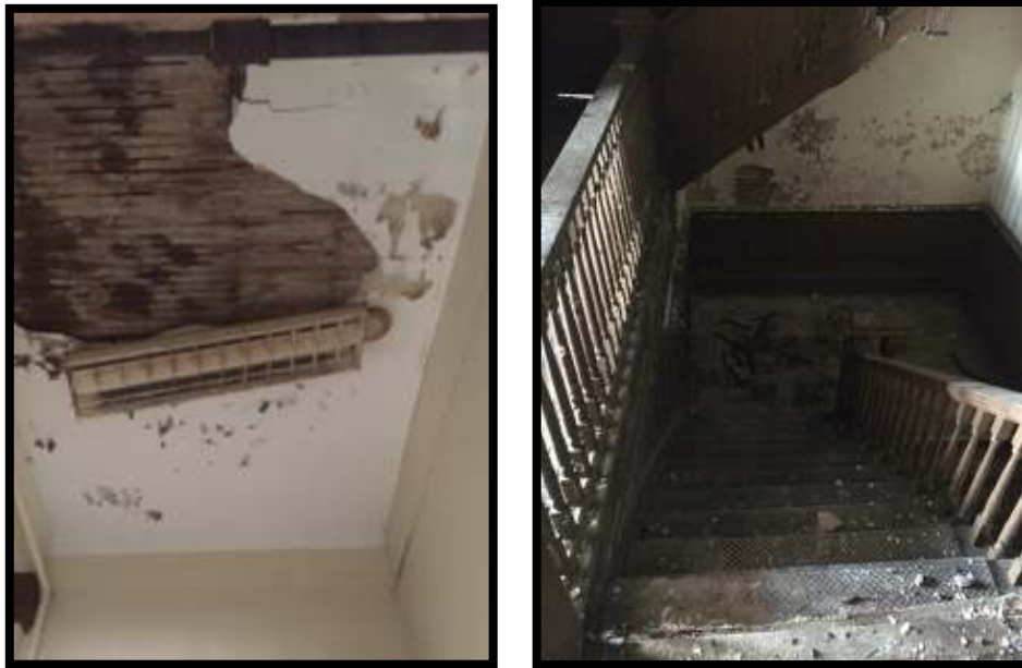
(L) Plaster ceiling damage (R) Water damage to wall plaster paint
