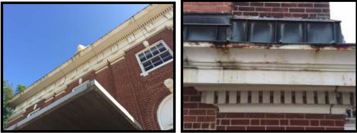
(L) View of cornice sections (R) Metal Cornice showing corrosion and copper top
