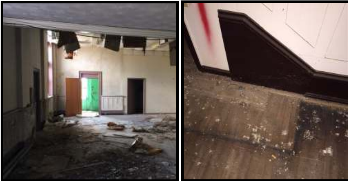
(L) Trim and Wainscot in Auditorium (R) Outline of missing steps and stage
